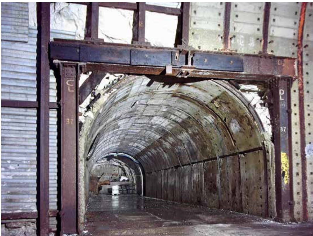
One of the large tunnels in the underground combined headquarters at Fort Southwick. Photo Adrian Armishaw
